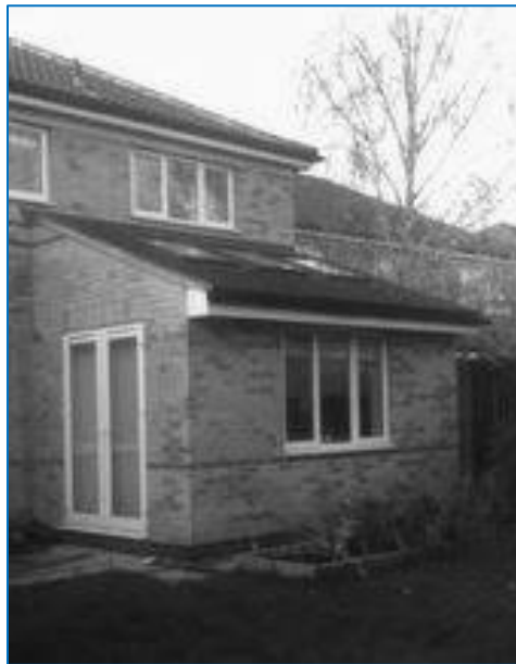
Figure 1: External wall of a house showing a 1.5 m projected triple glazed window.
